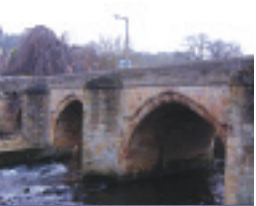
The downstream side of Matlock Bridge, as seen from the viewing area
